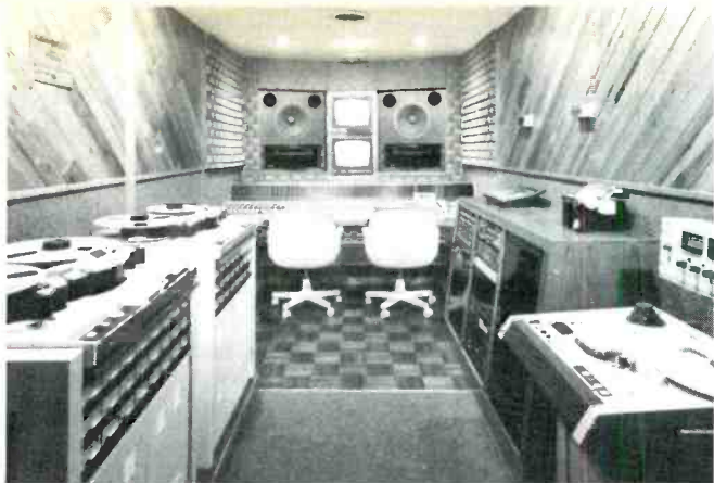
Mobile Audio truck's control room features Panasonic video monitors and Fostex audio monitors.
