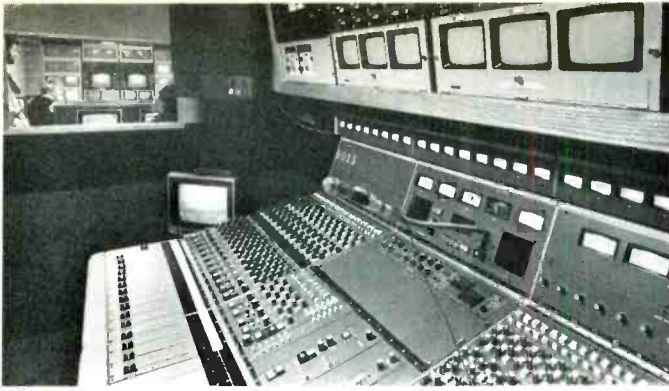
Inside Encore's spacious audio room. Control room is visible through window at left.
